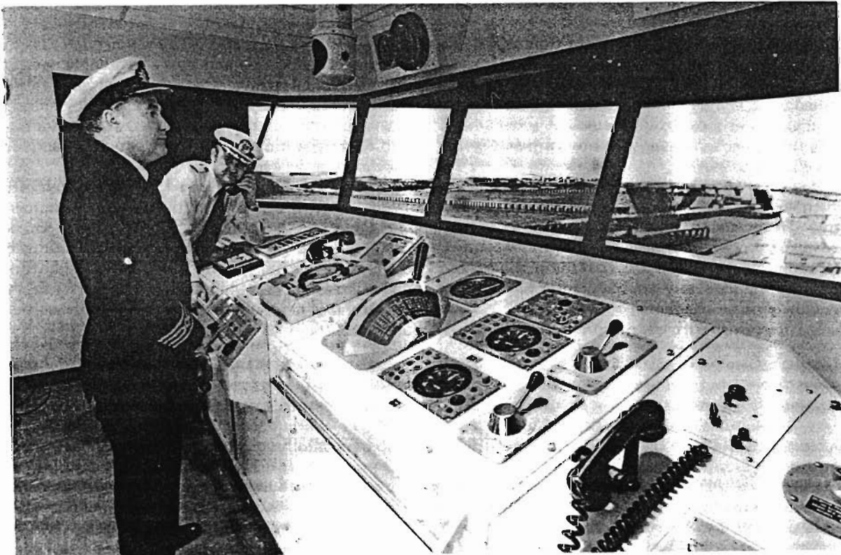
Fig. 40 Bridge console with steering, main propulsion, and thruster control
