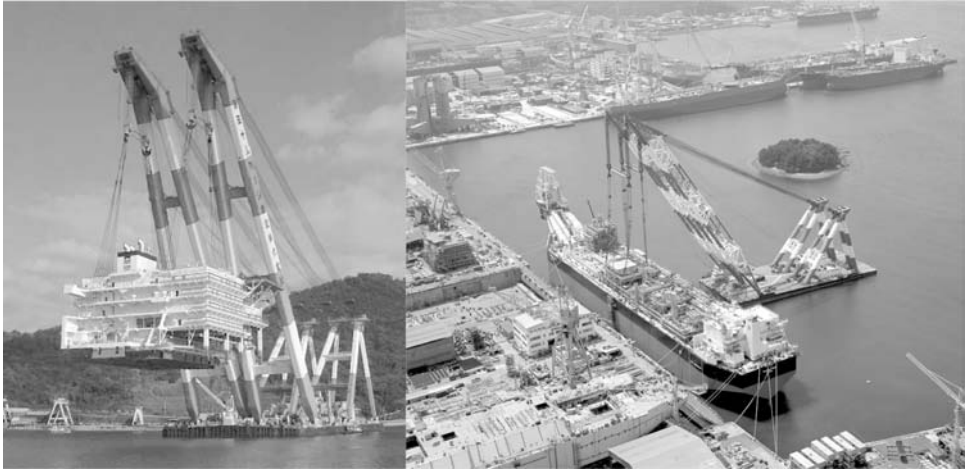
Figure 9.5. An assembly of large PAUs by heavy lift; for accommodations (left) and topsides facilities (right) (courtesy of Samsung Heavy Industries).
