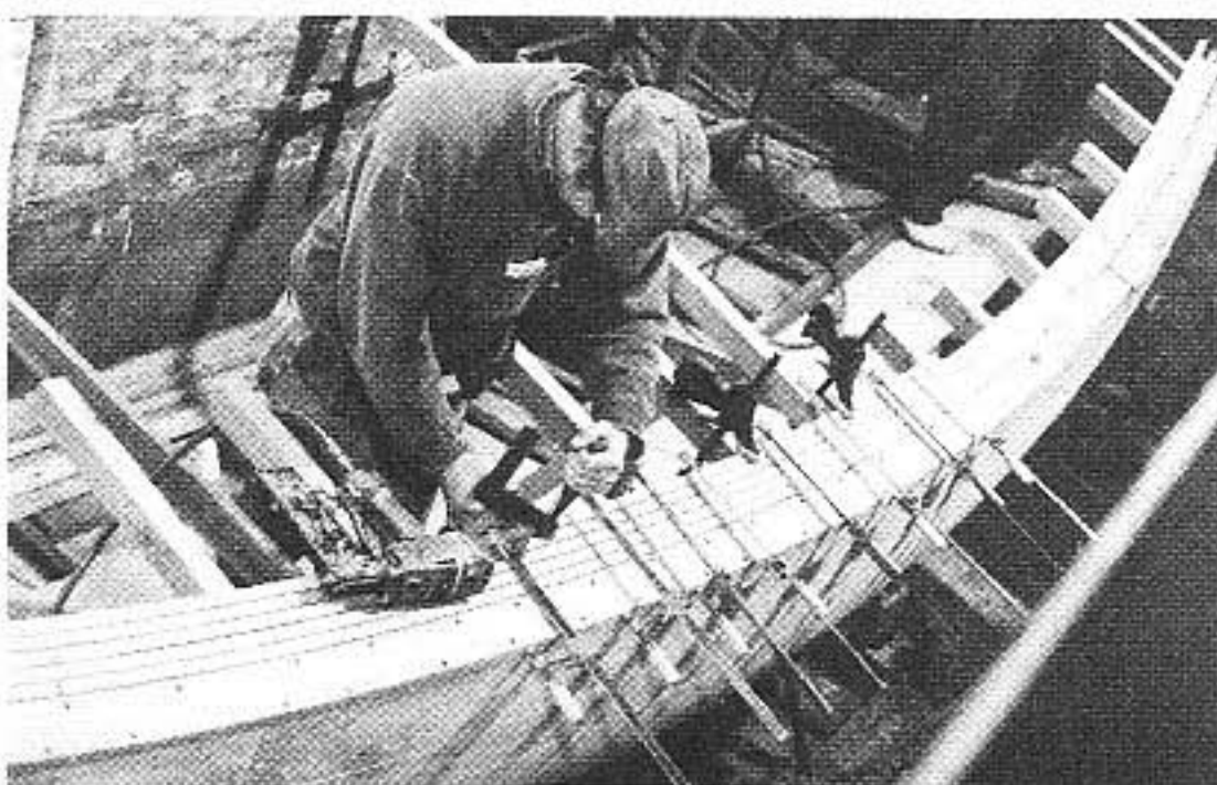
A laid-pine deck. Each strake is edge-nailed to its neighbor and toe-nailed into the deck beam below. A bead of 3M-5200 is between each plank. (Courtesy Kortchmar & Willner)
